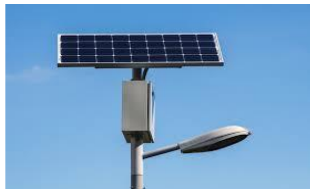
Fig. 3 Street light based on Solar System
