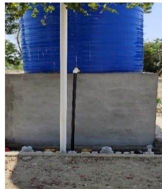
Fig. Main supply Tank
