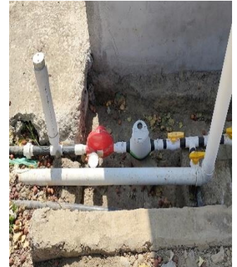
Fig. Water consumption meter
