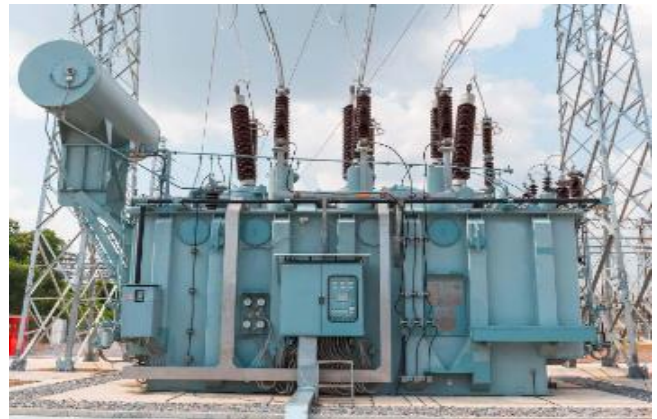
Fig. 2 Power Transformer at Grid Station
